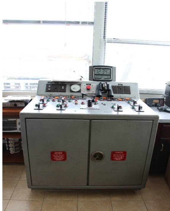
Condition Photo 10: Control panel in the operator's house.
