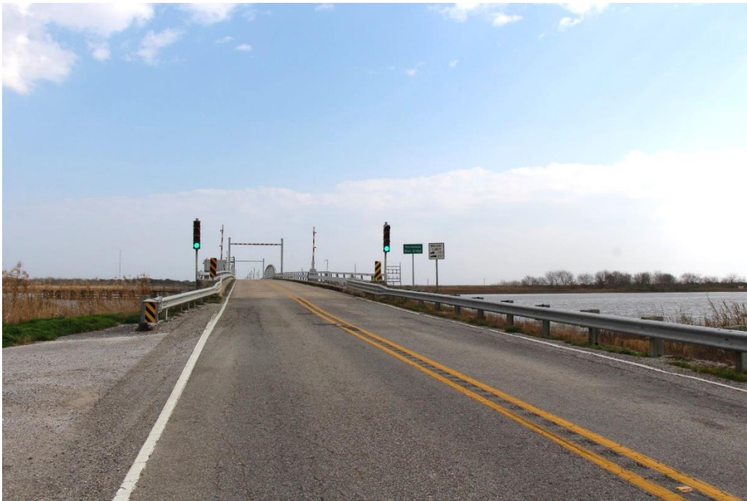
Condition Photo 14: West approach spans and west approach roadway with traffic signals and guardrail, looking east.
