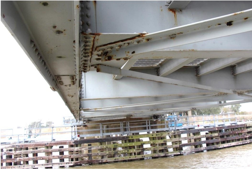
Condition Photo 5: Underside of truss span and floor system, showing paint system failure and rust at truss member connections.
