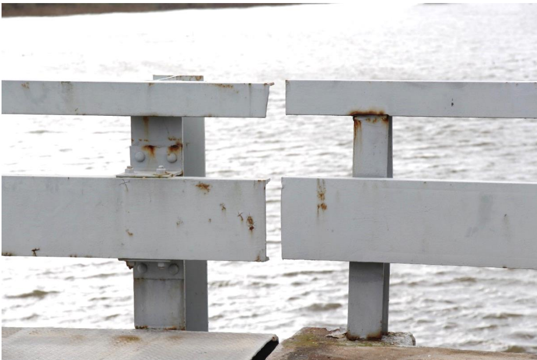
Condition Photo 6: Bridge railing rust and paint system failure, typical throughout the bridge. Photo at joint between approach span and swing truss span.
