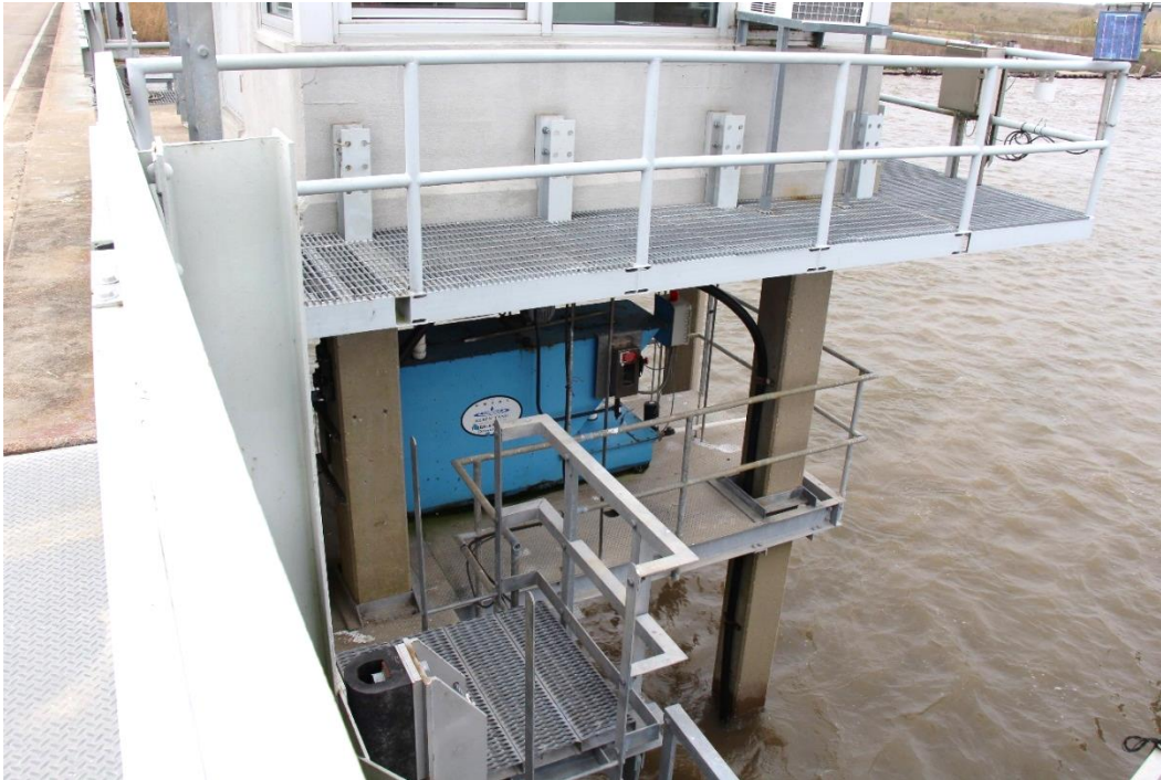
Condition Photo 9: Air compressor and sewage system under the operator's house.
