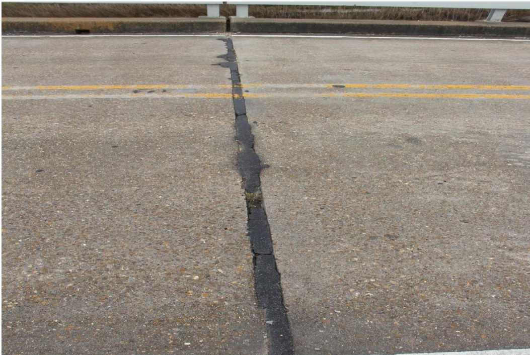
Condition Photo 2: Typical pour seal joint deterioration and vegetation growth in approach spans concrete decks.
