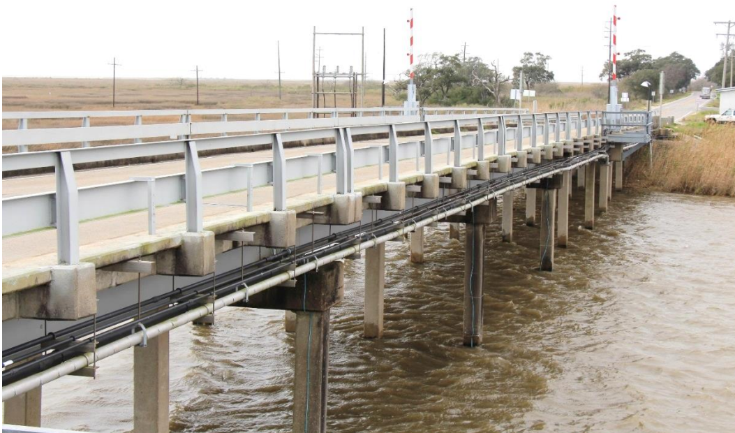
Historic Fabric Photo 2: Approach spans on either side of the main swing span and steel railing.
