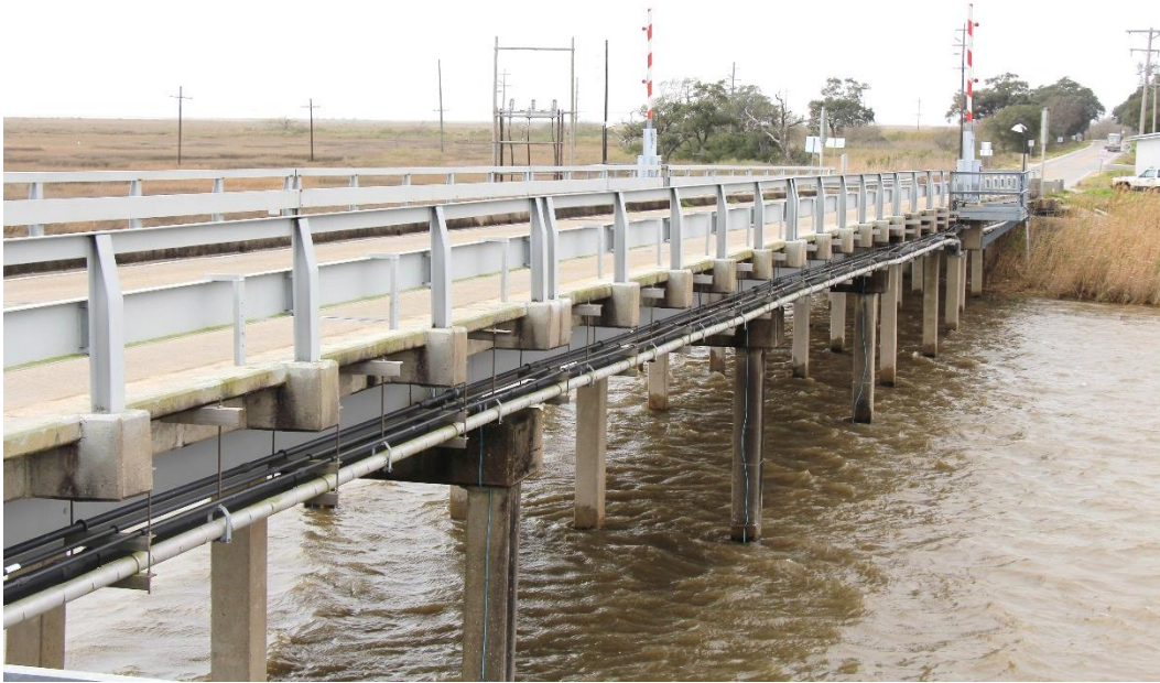
Condition Photo 17: Discoloration of the approach west span bents.
