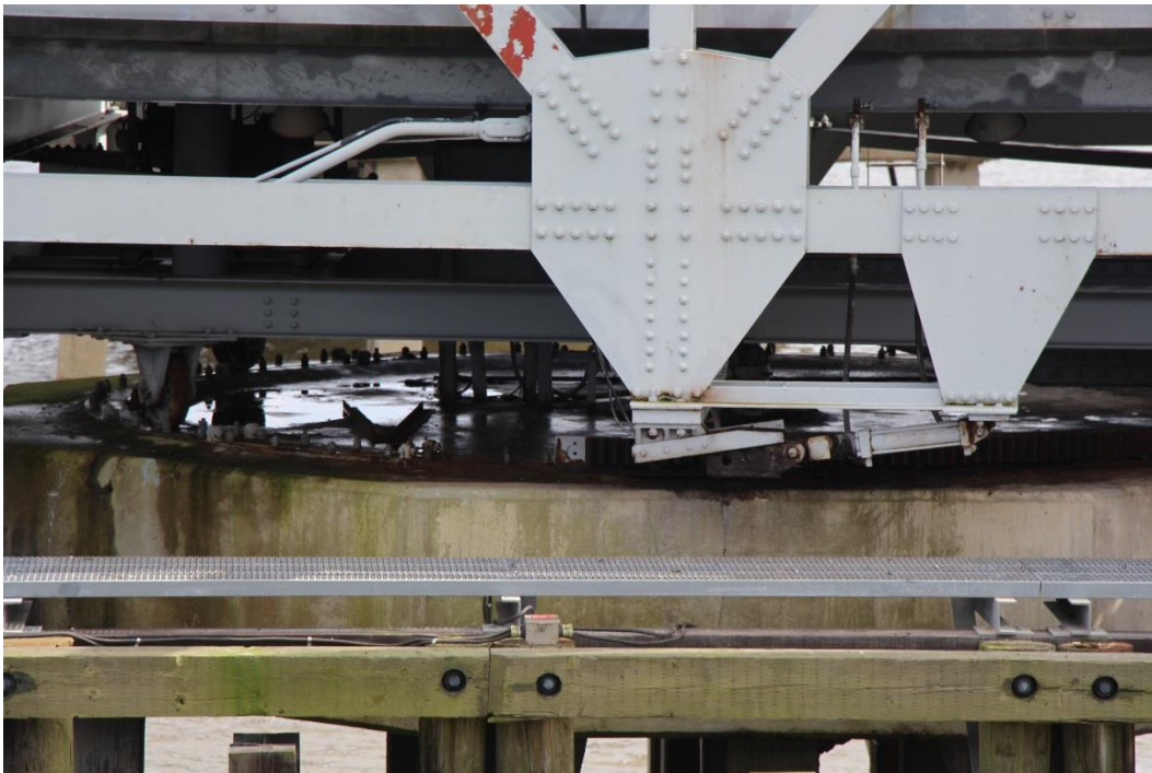
Condition Photo 18: Center concrete pivot pier with operating machinery, center pivot bearing, and pivot rail and rollers.
