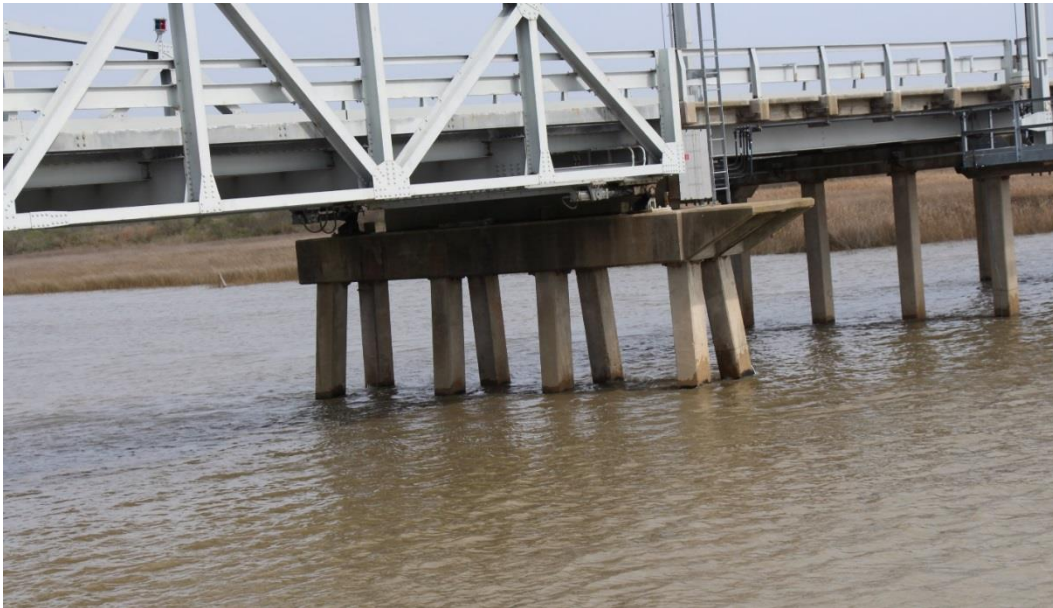
Historic Fabric Photo 1: Substructure and approach spans, typical of each end of the swing span.
