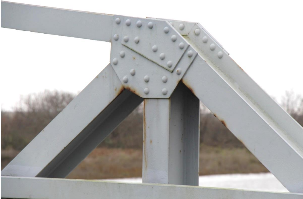
Condition Photo 4: Paint system failure and rust at pony truss connections; upper chord connection joint shown, other connection joints similar condition.
