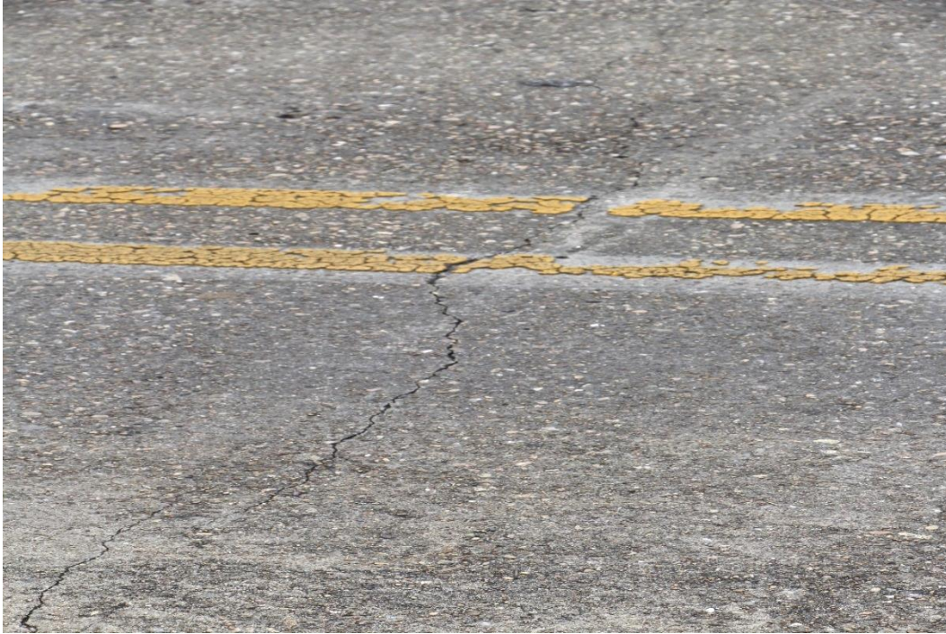
Condition Photo 3: Typical cracking in top of concrete approach spans, longitudinal cracking, and painted lane line striping faded.
